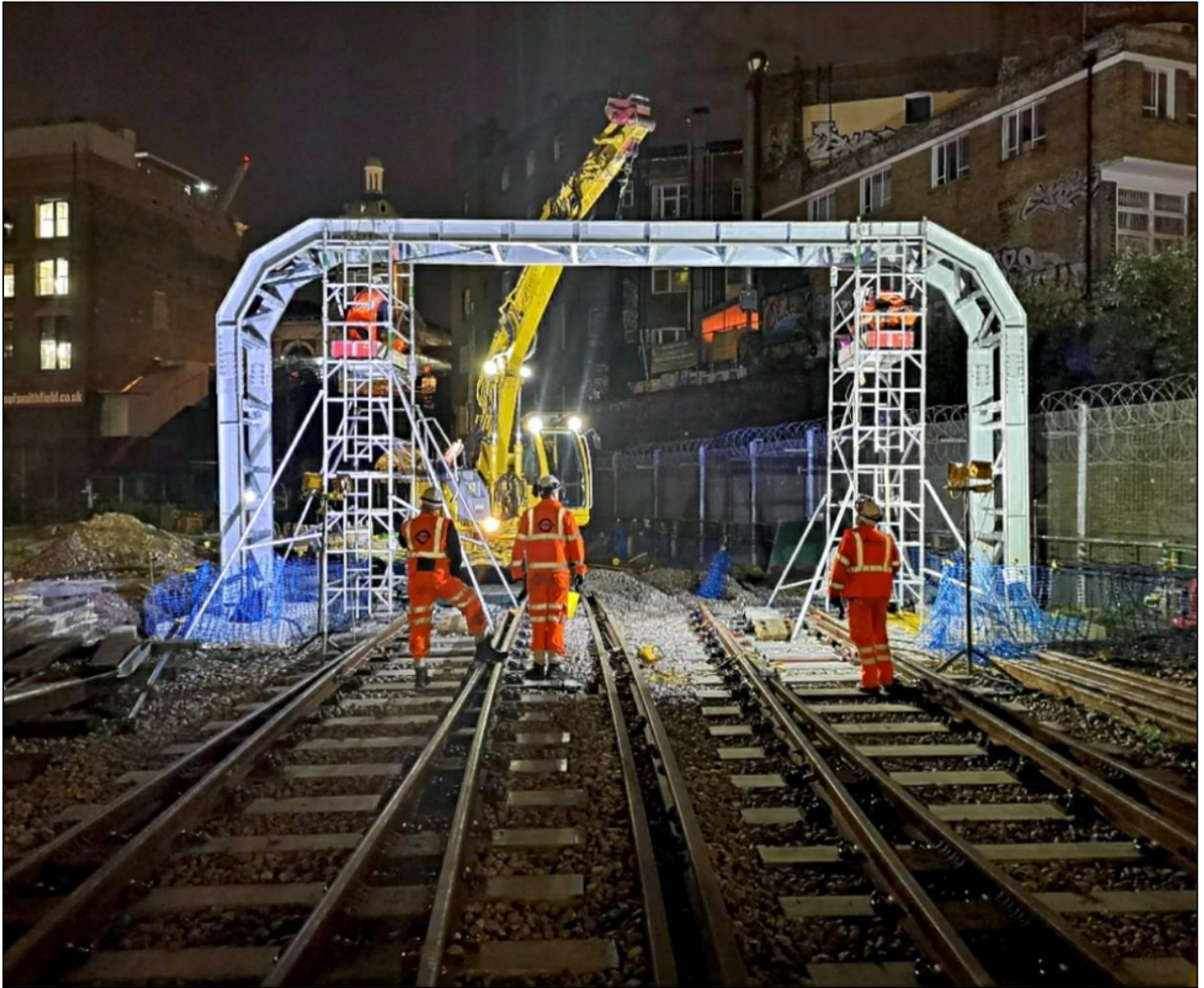
Above: During non-traffic hours on 2/3 September 2018, a cross member was added to complete the new over track crossing at the entrance to the future Farringdon City Sidings.
